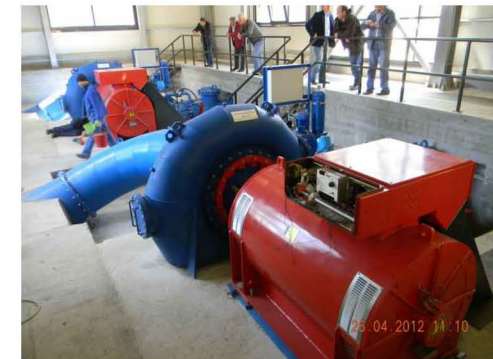
HPP Sadu A Machine hall
