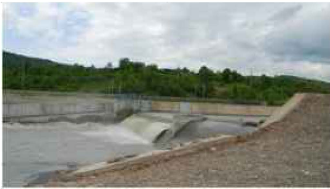
Water intake Breaza on Prahova River.
